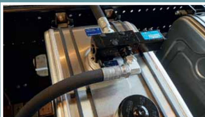
Tipping valve mounted on the return filter
