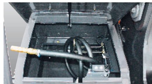
Electric fuel refilling pump
